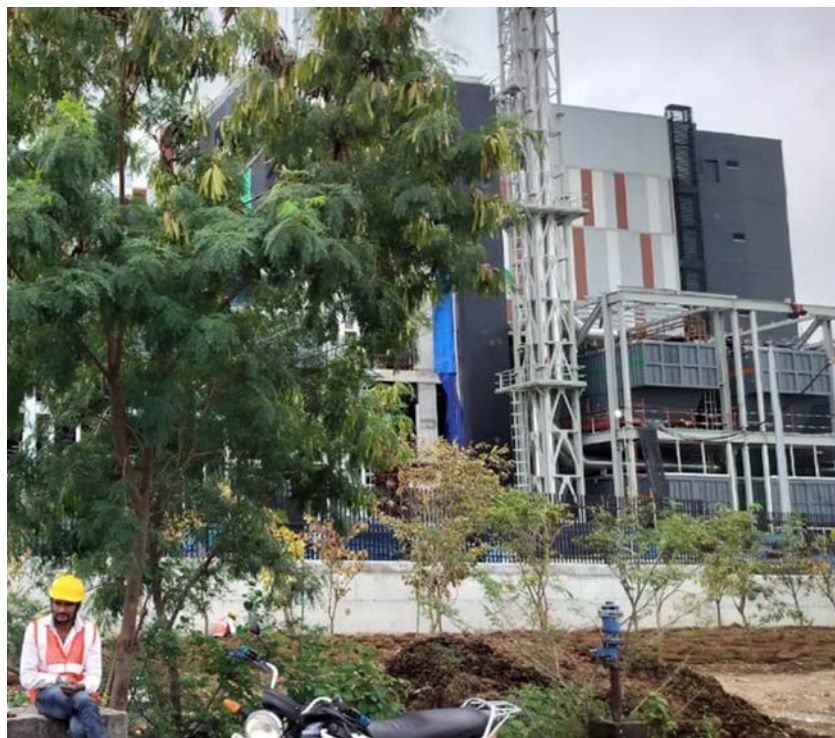
Microsoft Data Center, Mekaguda
